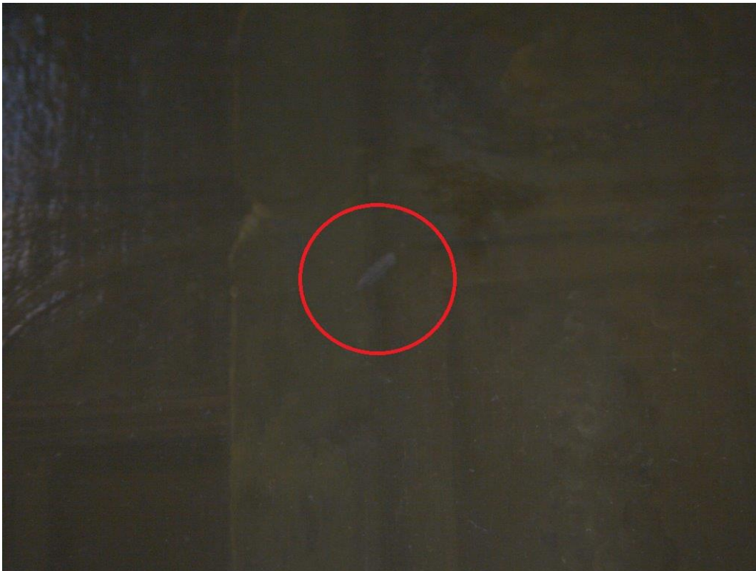
Figure 12: A problematic gash penetrating through the ground layer and into the panel itself.
